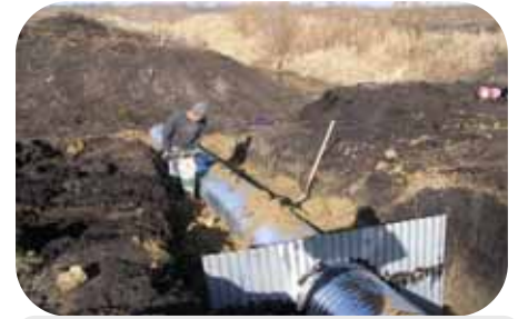
Side Inlet Pipe being installed to provide a stable outlet for a grass waterway.
