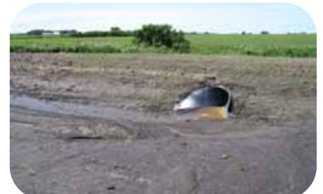
Side Inlet protecting an open ditch bank. Note water flowing through.
