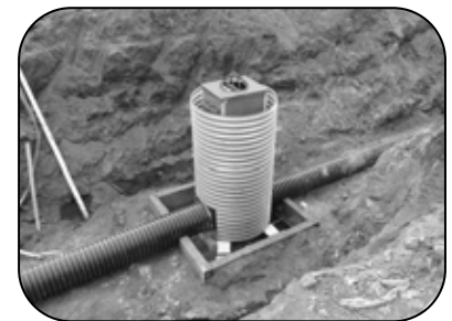
Structure to regulate water levels in a restored wetland
