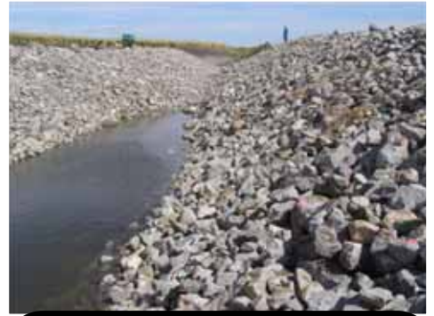
Rock Chute at Dale Stensrud site to stabilize the grade of the ditch in October 2014 using EQIP funding partnered with Freeborn County SWCD & GBERBA using Clean Water Funds
