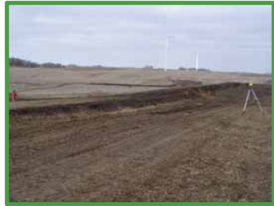
Staff completing a construction check after a water & sediment control basin is installed
