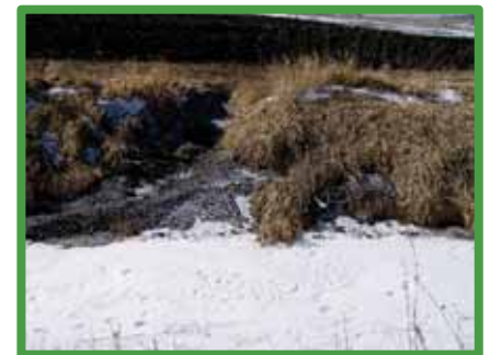
Sites like this gully entering a public water are eligible to apply for GBERBA funds
